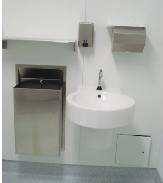
Hand basin facility at CSIRO
