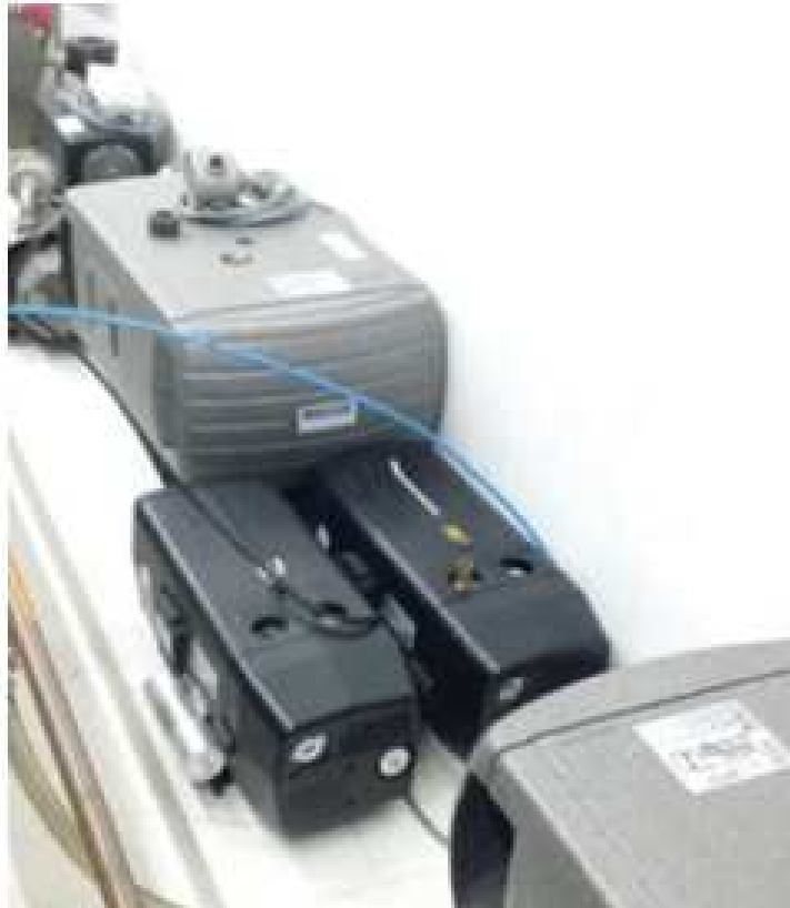
Individual vacuum pump install at production machine (40 units) . Noise level (90 dB)
