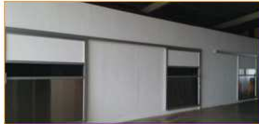
Installation of centralize vacuum pump at facilities plant building complete with noise absorption material (rockwool with cement board). Noise level reduce to avg < 70 dB
